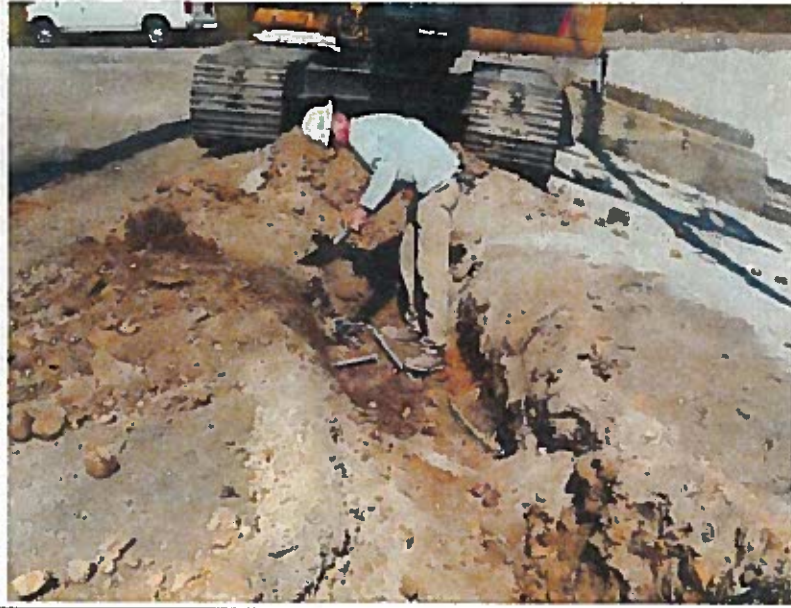
Hand exposing damaged utility south of the North Concrete Inlet Structure
