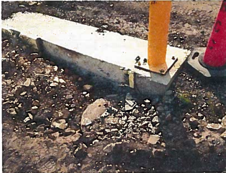
View of Sampling Building upslope cylindrical foundations near rectangular concrete pad, facing south
