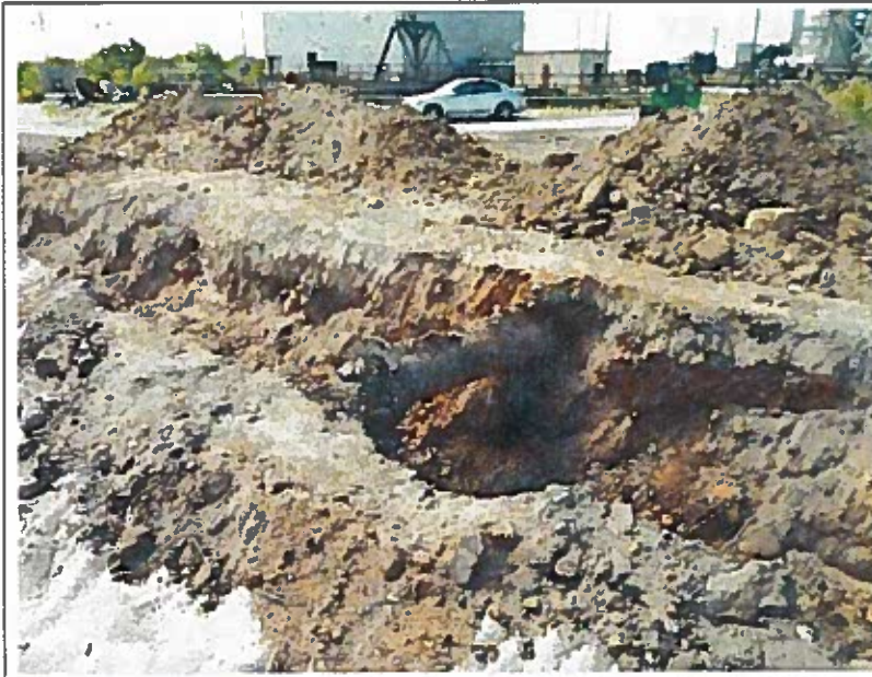
Abandoned 8 inch diameter pipe near the North Concrete Inlet Structure, looking south
